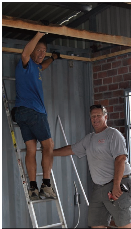
PAUL GETZ AND MARTY GOTTSCHLING rough wiring for a new school building.
