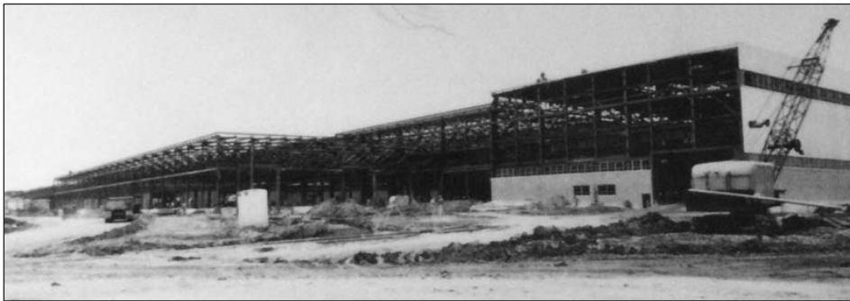
ALMOST ALL STEEL had been erected, which shows the beginning of outside brick work and siding
