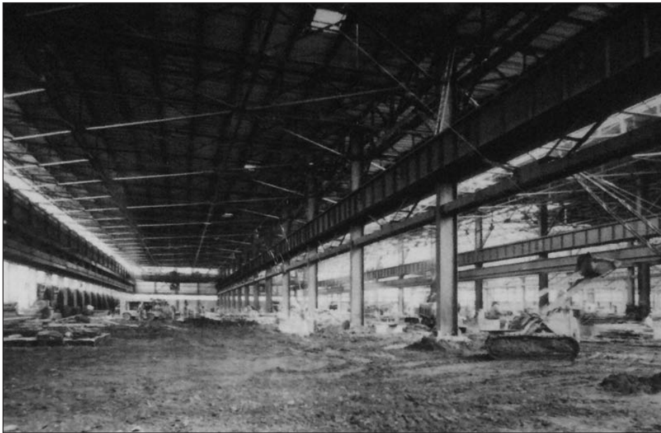
NO CONCRETE floors had yet been poured when these photos were made by Jeff Sprang in 1956.
