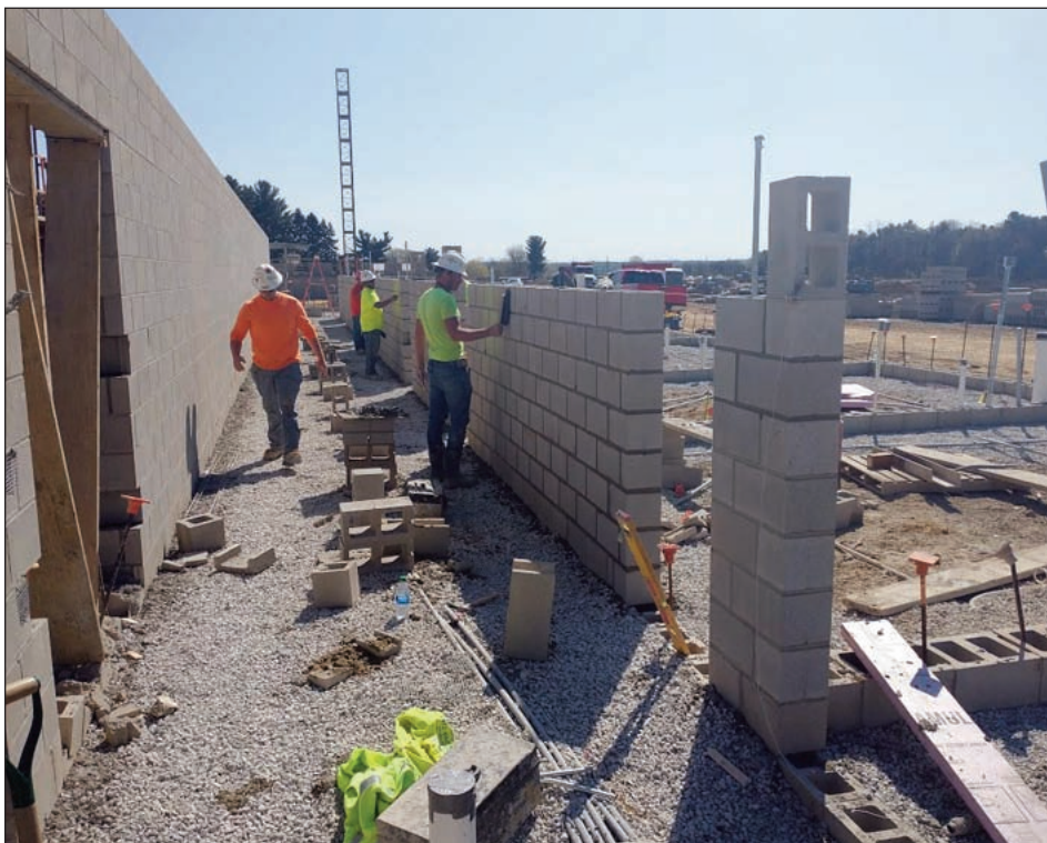
CONSTRUCTION on the Lexington 7-12 building project continues. The crews made nice progress the last month.
